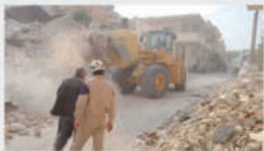
Emergency responders clear rubble with Syria Regional Program-provided heavy machinery following a regime attack in Hama, Idlib, in November 2014.
