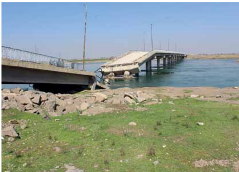
Bridge in Muqla Qabira village, Raqqa Governorate, demolished in a US-led Coalition air strike. Photo by volunteers of the Foundation for the Study of Democracy
