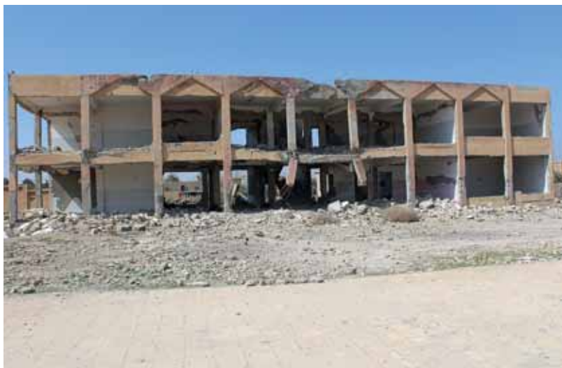
Ganem Al-Ali village school in Raqqa Governorate demolished in a US-led Coalition air strike. Photo by volunteers of the Foundation for the Study of Democracy
