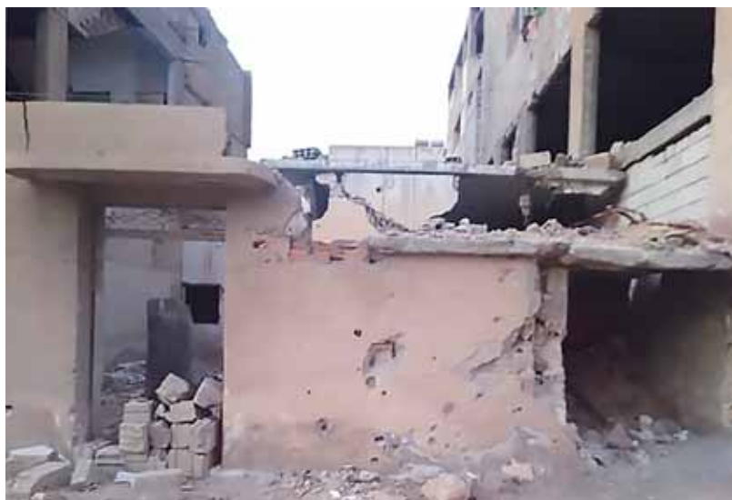
House of Taga Al-Musa Halaf, 45, Raqqa, Raqqa Governorate, destroyed in a US-led coalition air strike in July 2017. Photo credit: Taga Al-Musa Halaf
