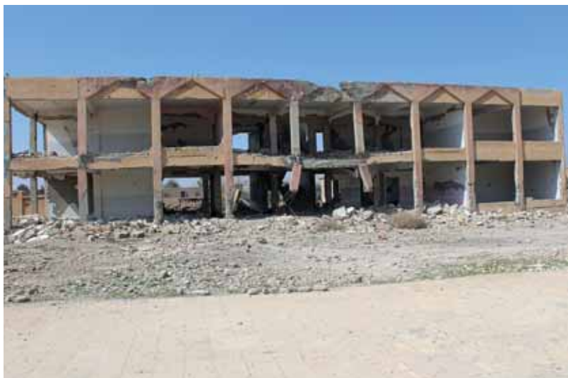
A school in the village of Ghanim al-Ali, Raqqa governorate, destroyed in an air strike by the US coalition. Photographs: volunteers of the Foundation for the Study of Democracy
