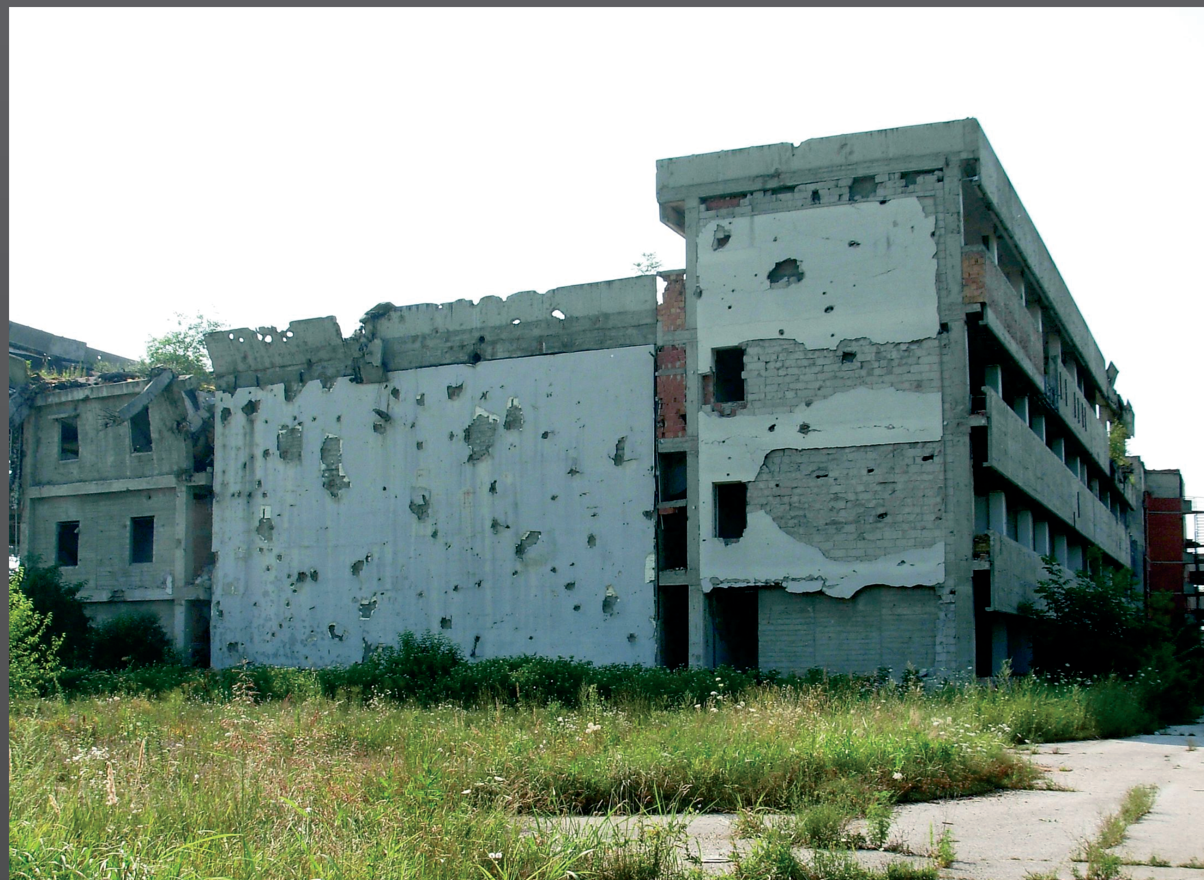
The building of the television channel in Mišeluk, destroyed by NATO bombing
